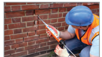
6. Re-point the mortar bed and make good the vertical crack with CrackBond TE3
